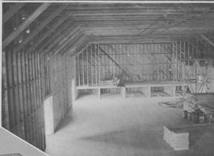
Below are two views of the new recreation hall, also built by Detachment Three. The top one portrays part of the stage under construction and much of the unfinished inside of the building.
