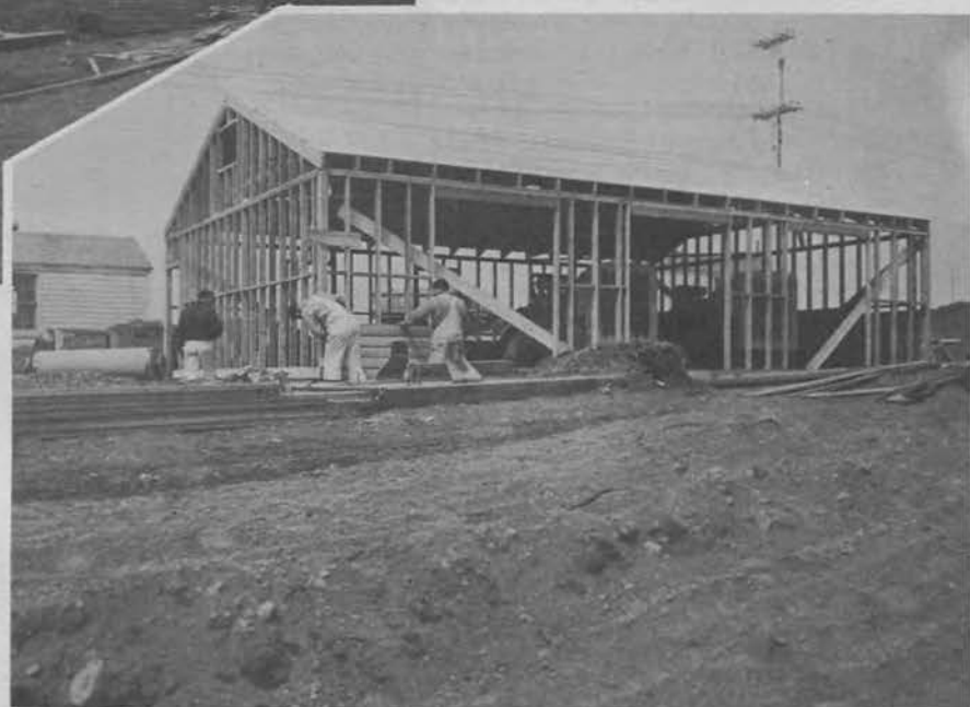
The two top pictures show two stages of construction on the generator building put up by Detachment Three at their Island X.
