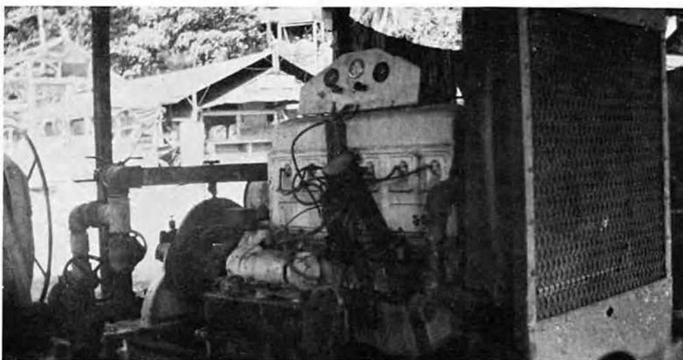
JAPANESE MOTOR USED TO OPERATE SALT WATER FIRE PUMP
