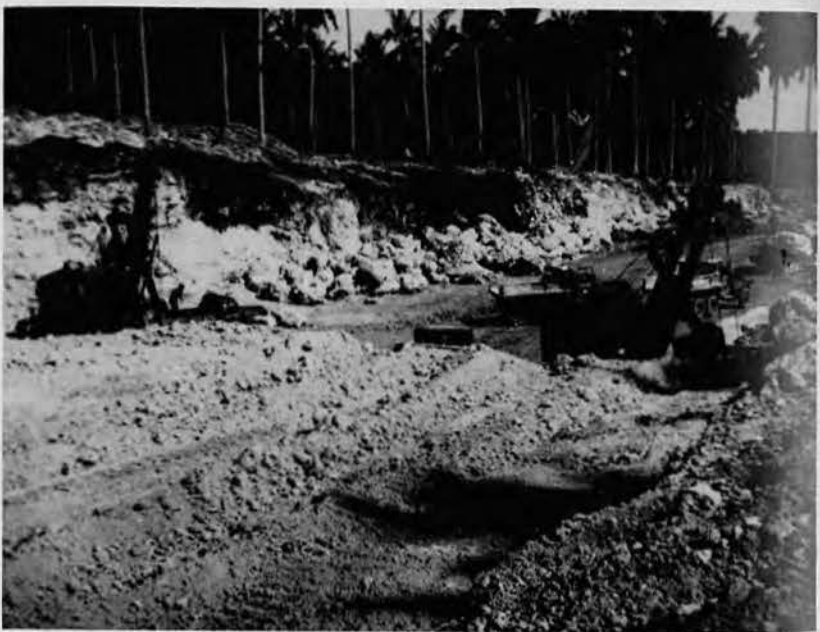
Top: Resurfacing section of island highway with coral. Bottom: Scene at one of coral pits.
