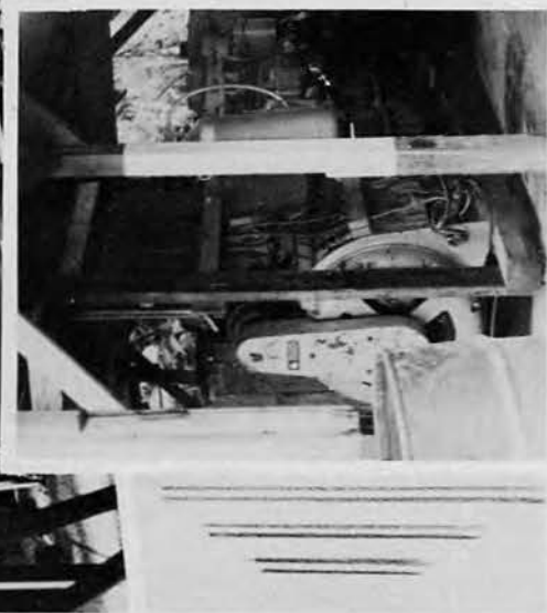
Center: General view of generator shed with electrical shop at left.
