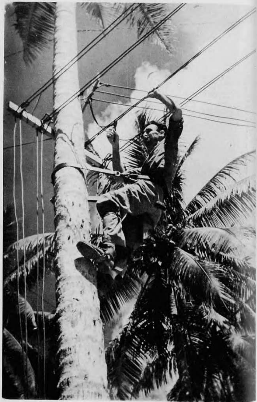
Unit electrical maintenance man splices tie into main line. Live coconut trees serve as poles.
