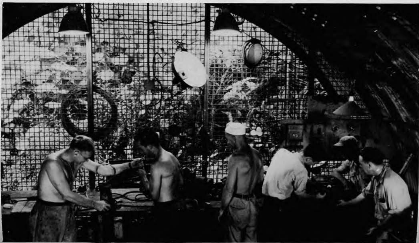
Quonset hut houses camp's electrical shop. Two men at left construct mounting for electric fan. Man at center tests motor armature while group at right makes adjustments on battery charger. Improvised test panel shows above them.
