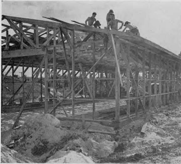
This warehouse was completed from the ground up in less than three weeks.
