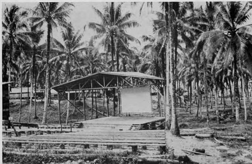
A shell of a stage had been constructed by the 44th Battalion.
