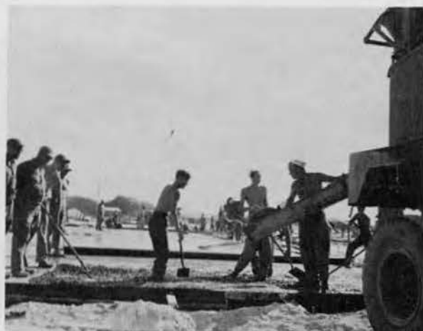
The concrete crew and the boys at the batching plant combined to turn out foundations and slabs in quantity.
