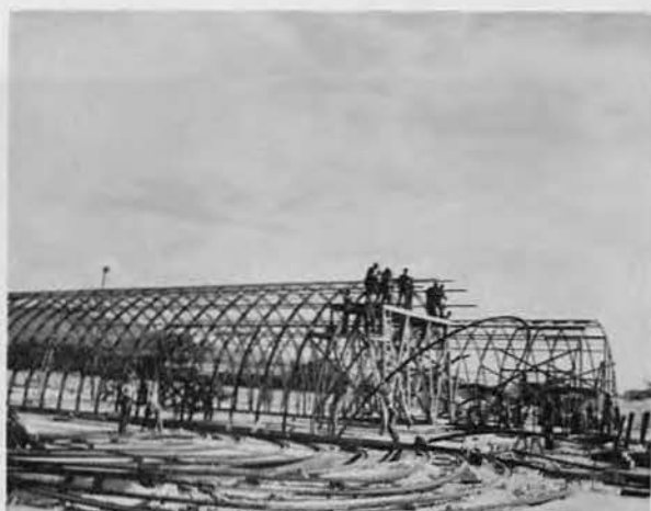
The old standby job was putting up big, pre-fabricated Quonset huts — B.O.Q.'s, WAVE barracks, shops and camp areas.
