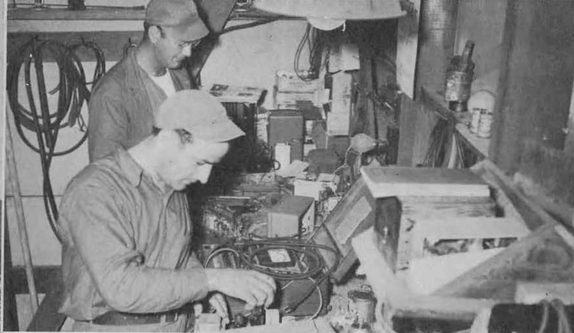
In the electric shop, permanent crews installed and kept operating vital electric facilities, power and communications. I. F. Dorman (rear) and John Berish check electrical equipment in the shop.
