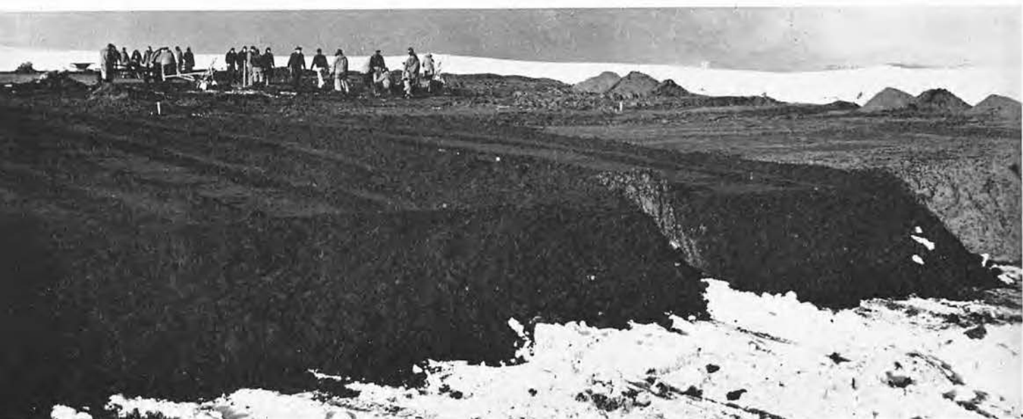
THE TEXTURE of wet sand made a nice photo after it was pushed and levelled by bulldozers. Men in the background are already laying the runway
