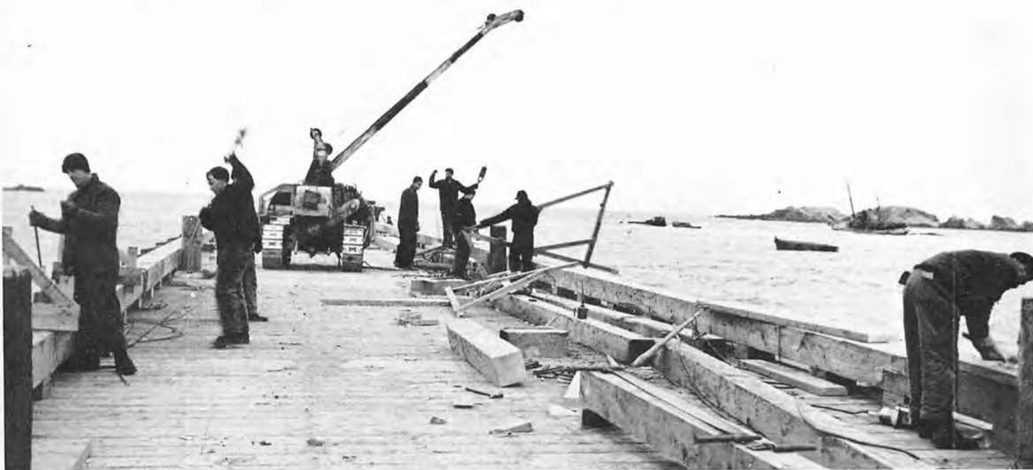
WIDE ENOUGH for two trucks to pass, the pier would speed the unloading of ships. A comparatively small number of us constructed this; most of
