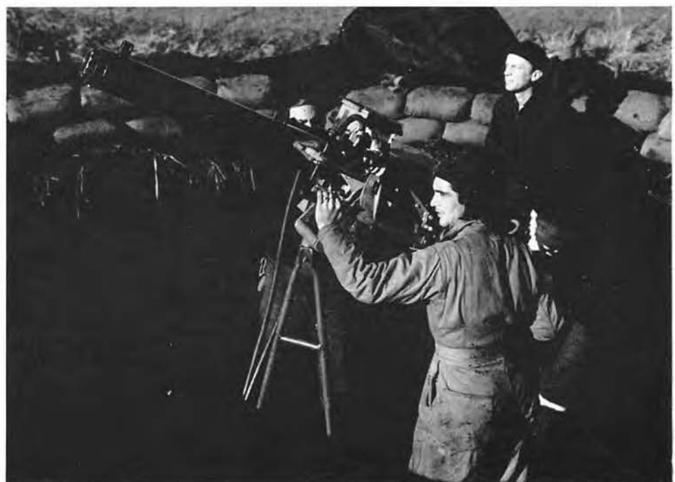
WE BUILT sand-bagged permanent gun emplacements, and some of us were selected as gun crews, ready to drop our tools and rush for a gun at a moment's notice.
