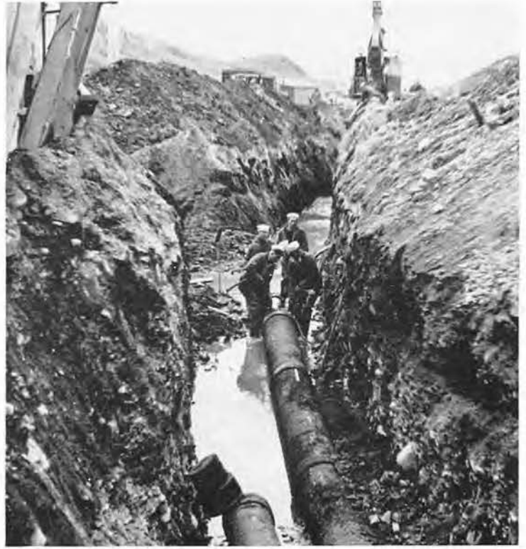
SECTIONS OF PIPE were fitted tightly by forcing a tapered end into the section directly behind it. A four-man battering ram furnished push needed.
