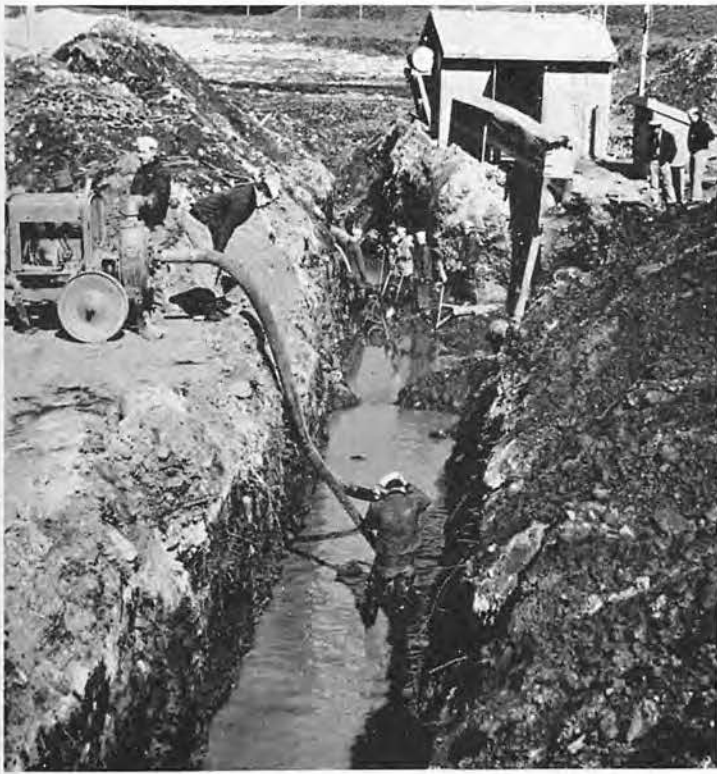
PERSISTENT RAINS, as well as surface drainage, sometimes kept our ditches filled with water. It couldn't be stopped, so we pumped it out instead.
