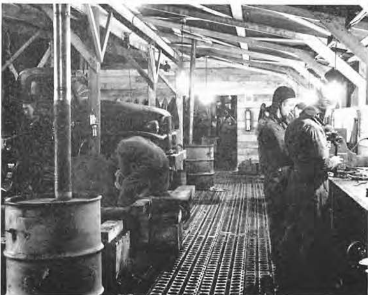
LATER, we built a garage into which trucks could be driven for repair under cover. We used runway mats for the floor.
