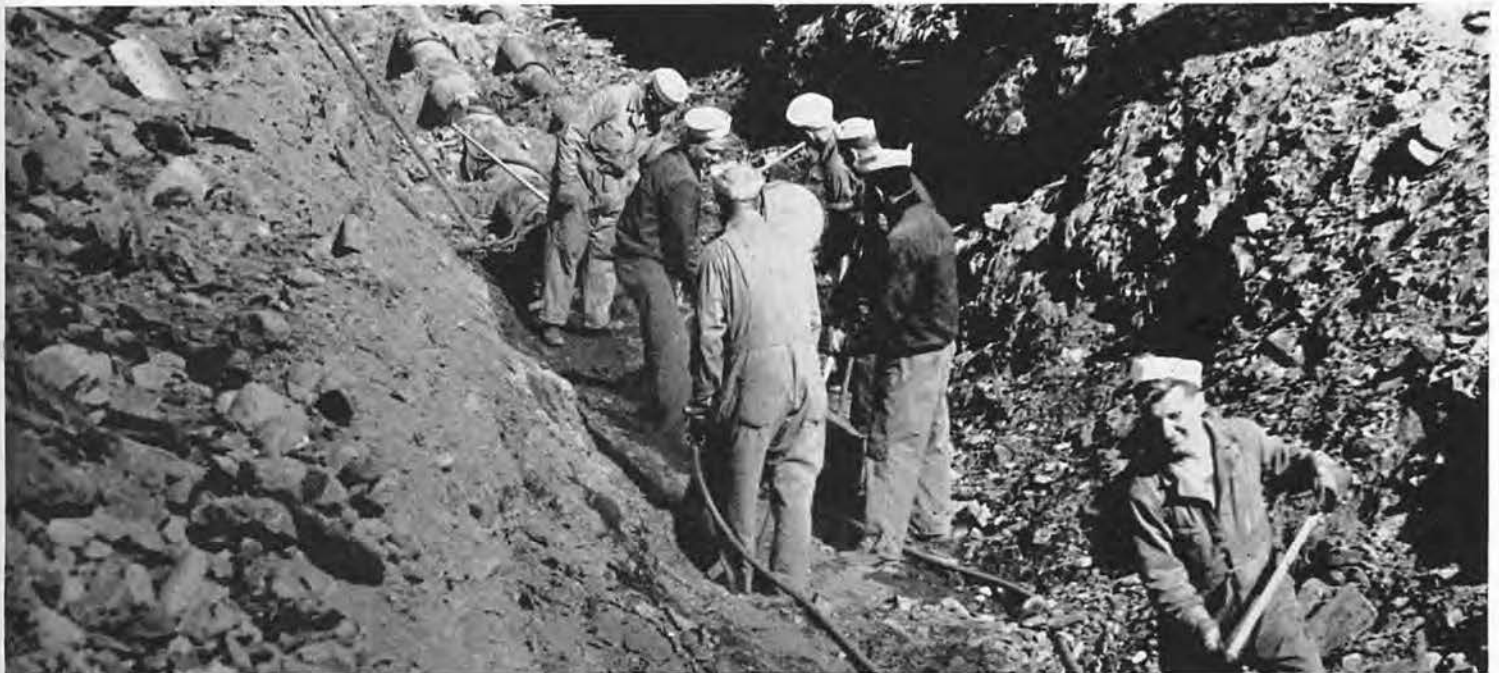
SOLID ROCK meant so much work with explosives and jack-hammers that the resulting ditch for a two-way parallel line assumed the proportions
