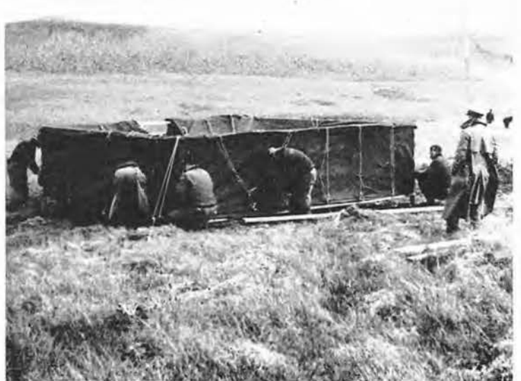
WE BUILT a two-by-four frame, four feet high, as sidewalls, before we put on the canvas. For a view of our finished camp in winter, turn the page.
