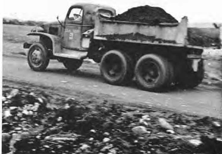
AFTER "floating" the sand and packing it down, we had hard surfaced, permanent roads, able to take a lot of punishment.
