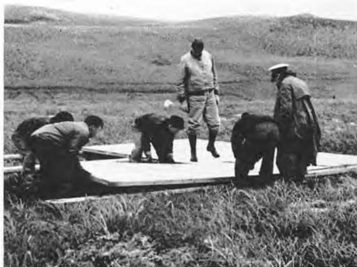
THE BOTTOMLESS tundra afforded nothing firm to support a foundation, but we did put in stakes and a few boards to brace the tent floors.
