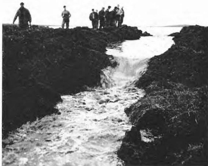
WATER GUSHED from a tundra lake as the last section of a drainage ditch was blasted.
