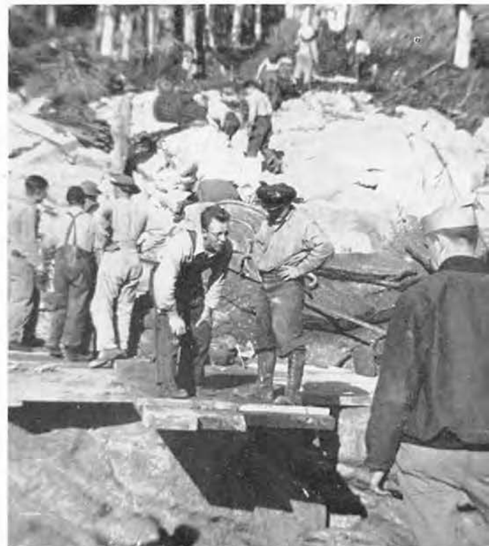
THIS FRONTIER COUNTRY gave us construction headaches. No small problems were the granite-hard rocks which covered almost every inch underfoot.
