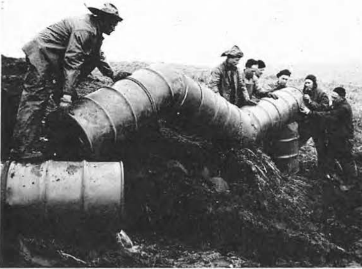
WE MADE OUR OWN sewer pipes, welding empty fuel drums together, and even throwing a few fancy curves. We made our own septic tank, too.
