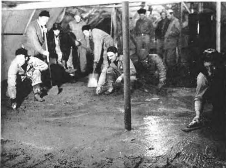
THE HEAD rated a concrete floor—or deck, if you insist. Head, sick bay, administration building and recreation hall were quonset huts.
