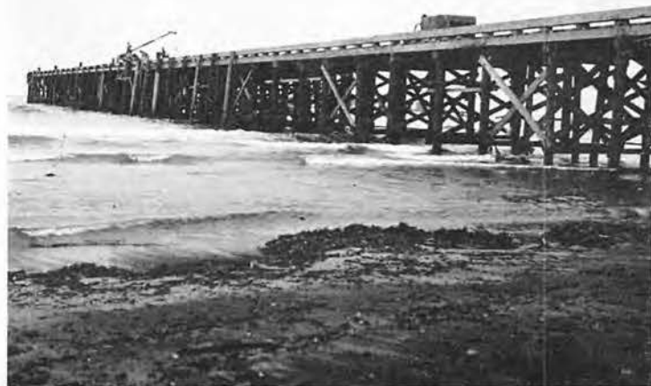
STOUT PILES, strongly braced, provided firm support for the pier, the last construction job we performed on the island
