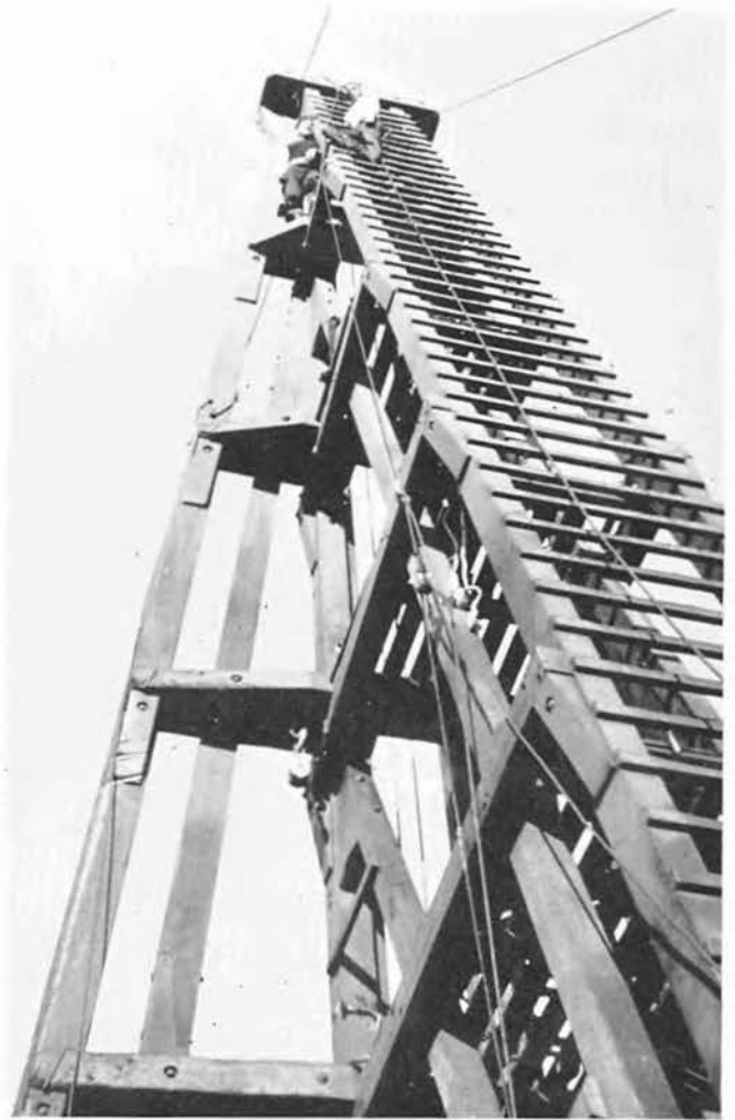
PERCHED HIGH ABOVE the water, we made frequent inspections and greasings of our pile-driver rig, keeping it ready for any job that might pop up without warning.
