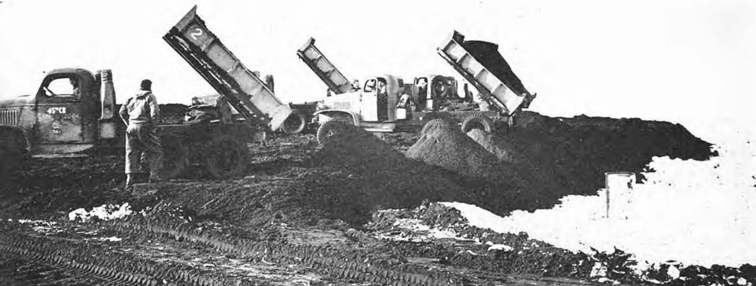
THREE, FOUR, sometimes half a dozen or more trucks were dumping at the same time. Some of us served as traffic cops, to direct the drivers to the
