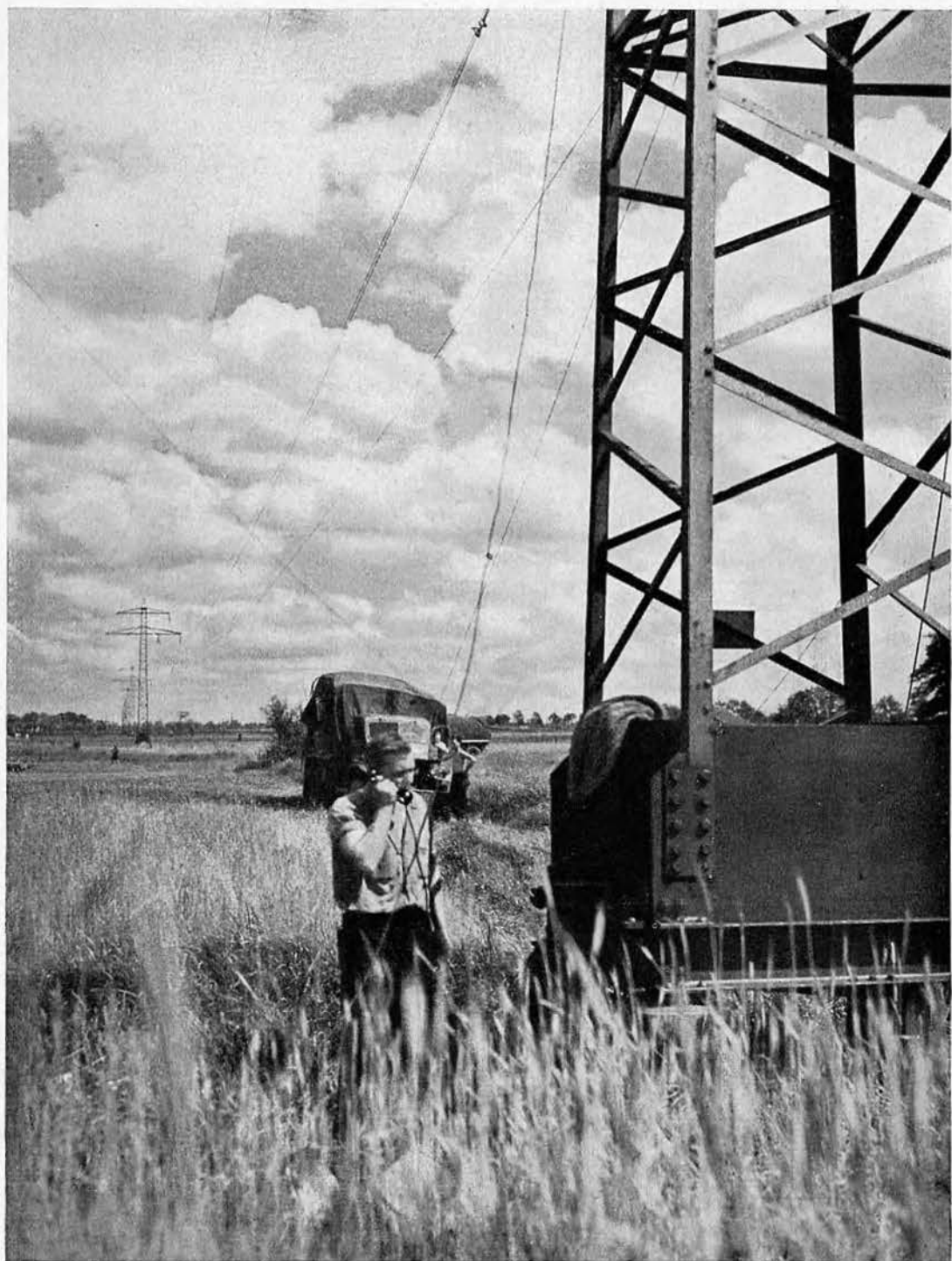
HIGH LINE CREW, suspending the high tension lines that are being restored to service.
