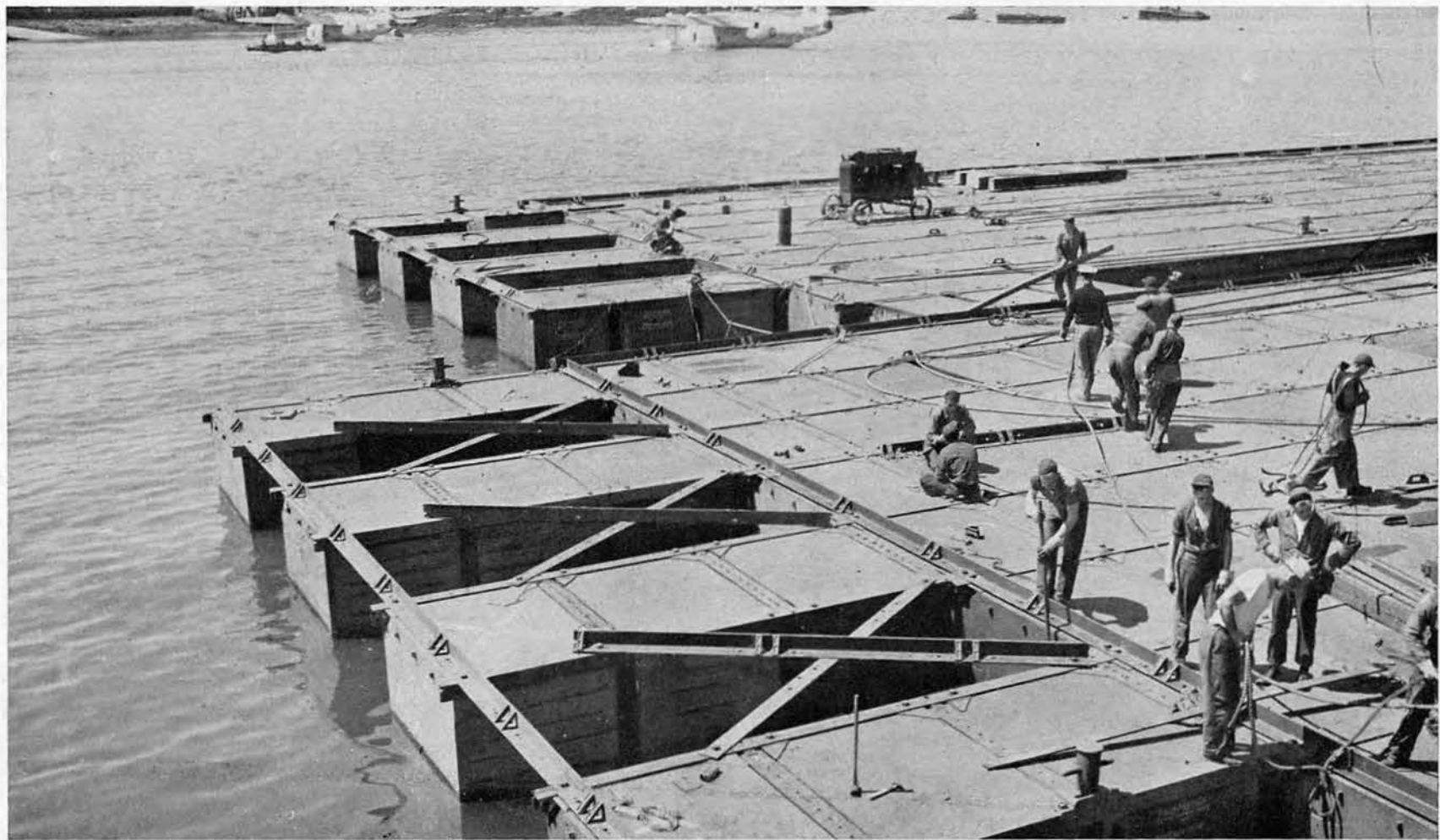
RETAINING CABLES: Laying out cables which, when clamped around entire tow, act as an additional security against "cracking up" in heavy seas.
