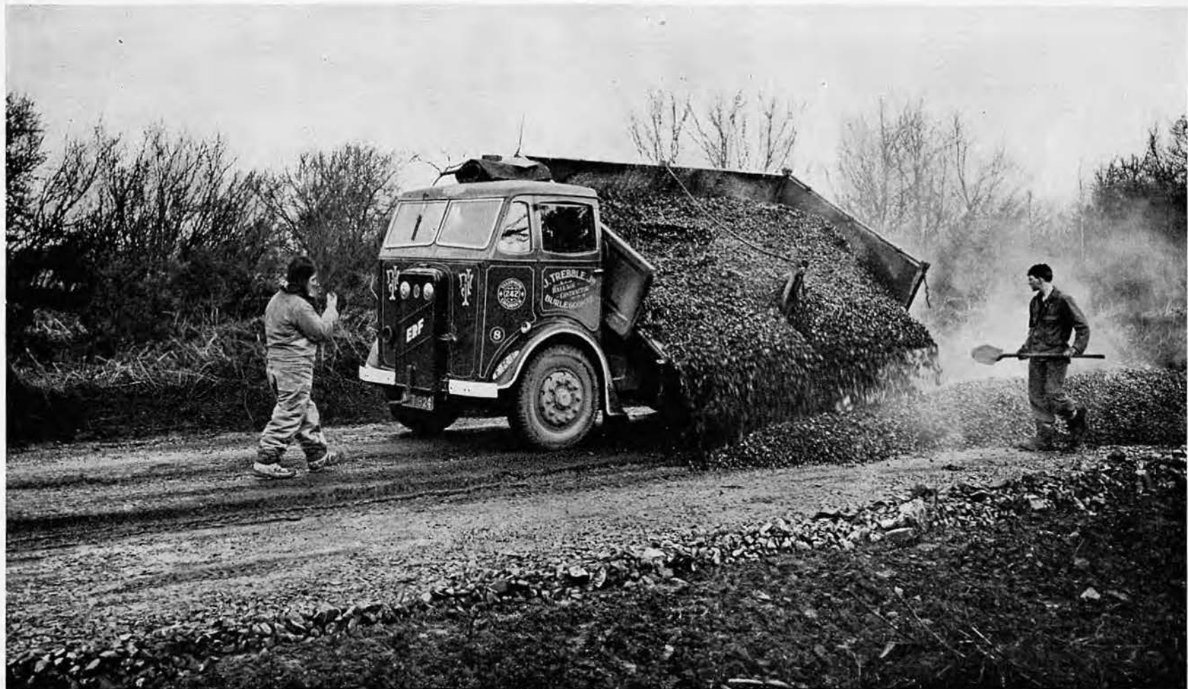
ROAD CONSTRUCTION: Laying the smoking "Tarmac" black topping on the road widening project between Dunkeswell and Upottery air fields near Taunton.
