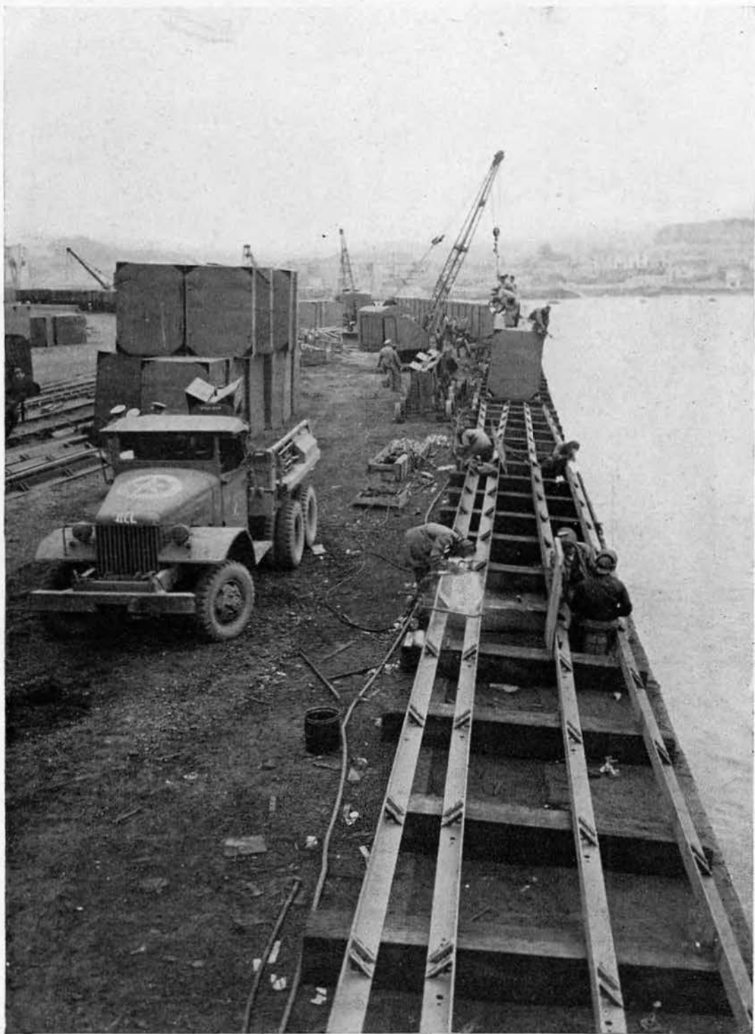
ARC WELDERS joining angles for long pontoon strings, to be used in the assembly of finger piers. A steel splint is welded across the abutting angles.
