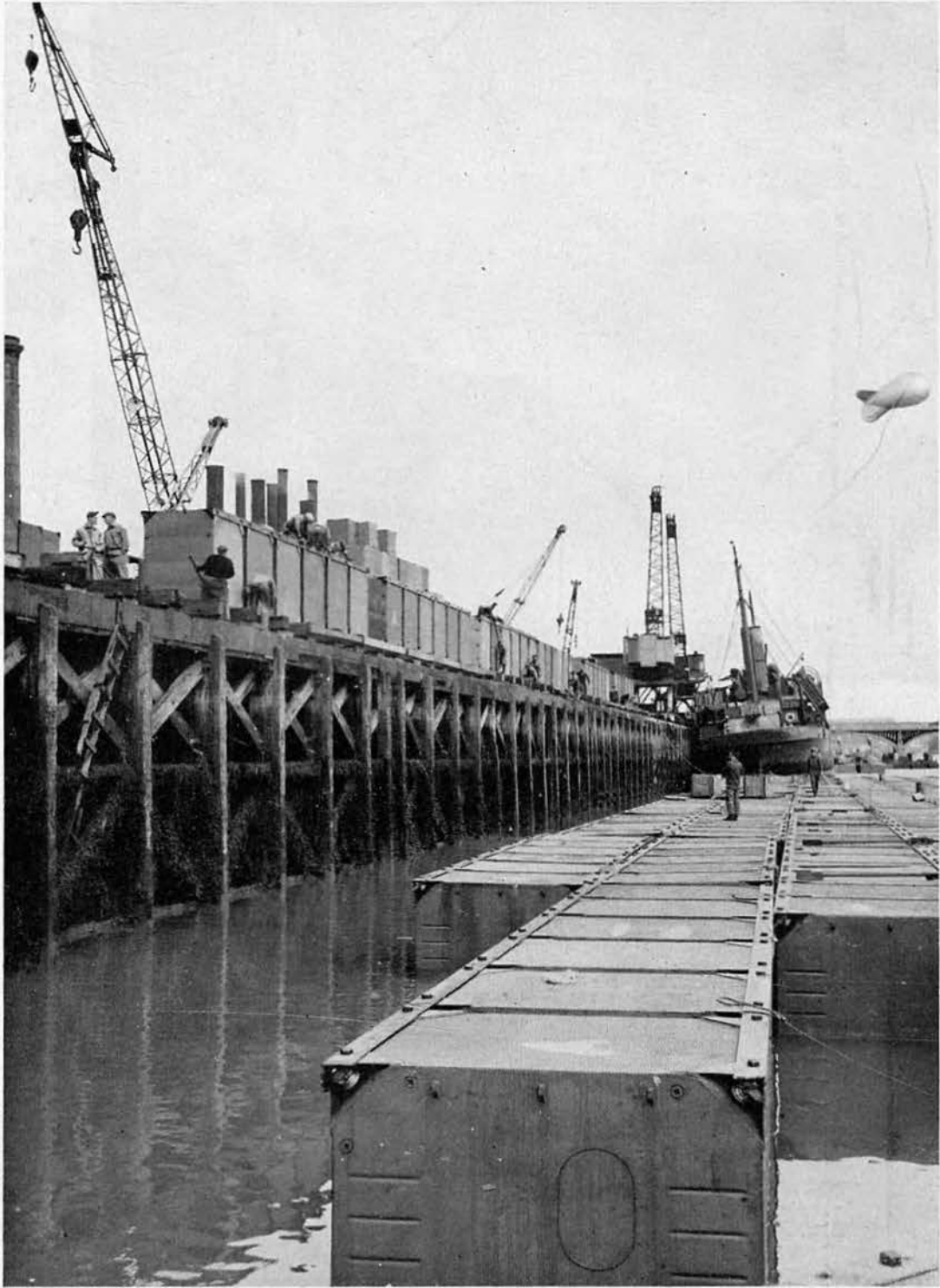
PONTOON STRINGS on the ways ready for launching. Tidal fluctuation here was approximately seventeen feet. Strings in the water are lashed together and anchored to prevent drifting until assembled into "tows".
