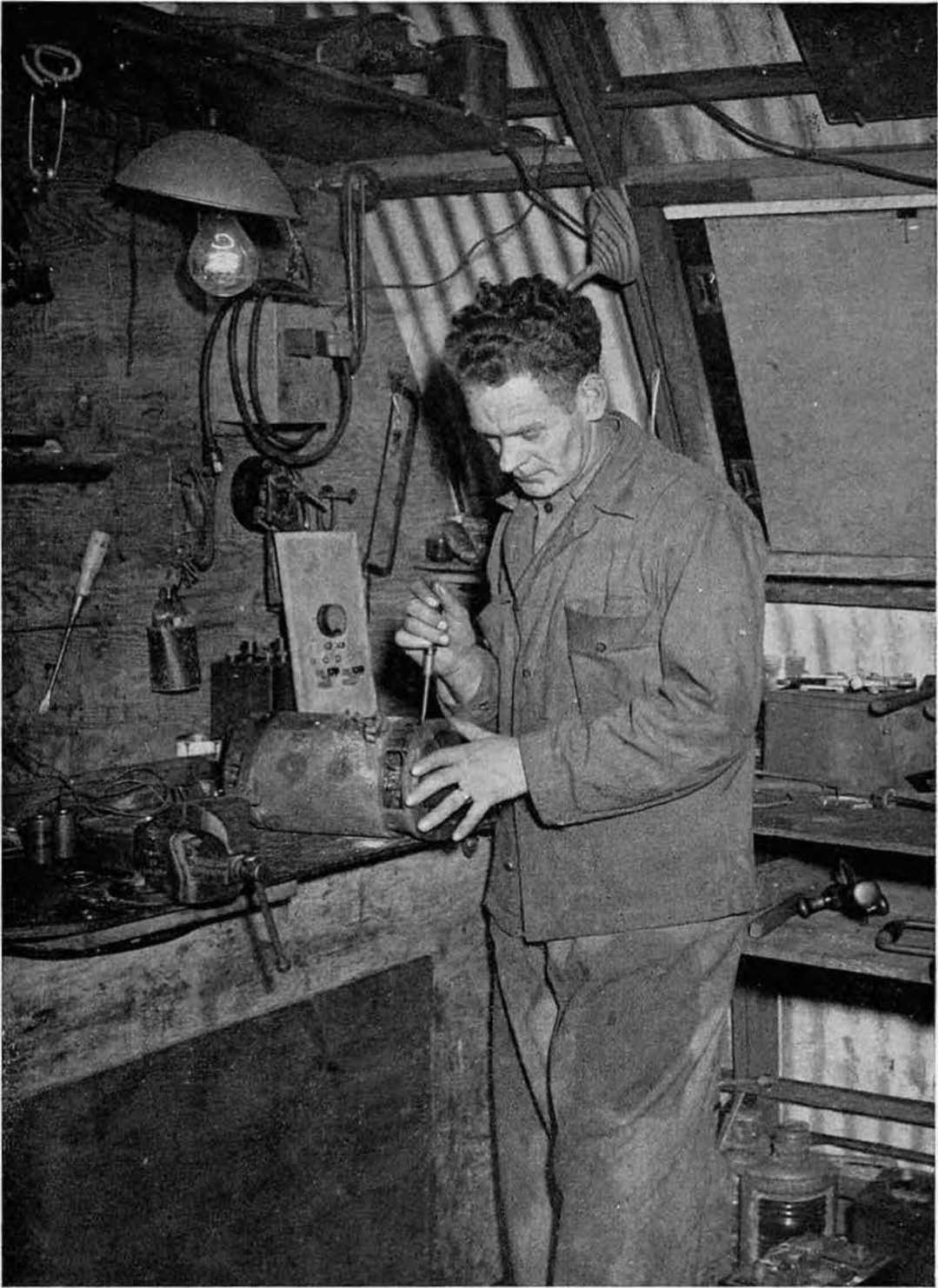
ELECTRICAL SHOP aboard the Rhino repair barge. A truck generator being repaired for an improvised battery charging apparatus.
