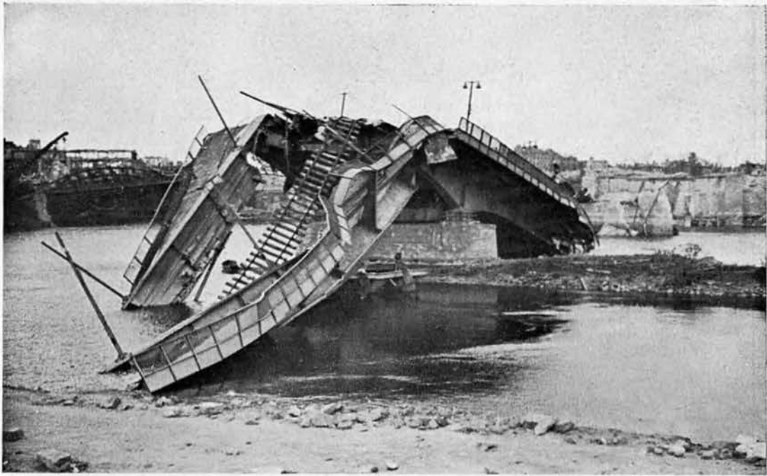
TWISTED HULK OF A BRIDGE across the River Weser at Bremen, Germany.
