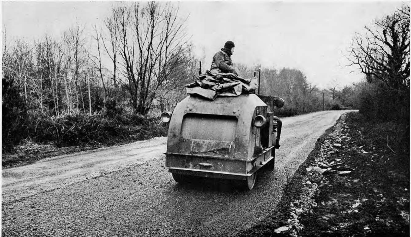
ROLLING THE STRIP to compact the substance and complete the paving operations.
