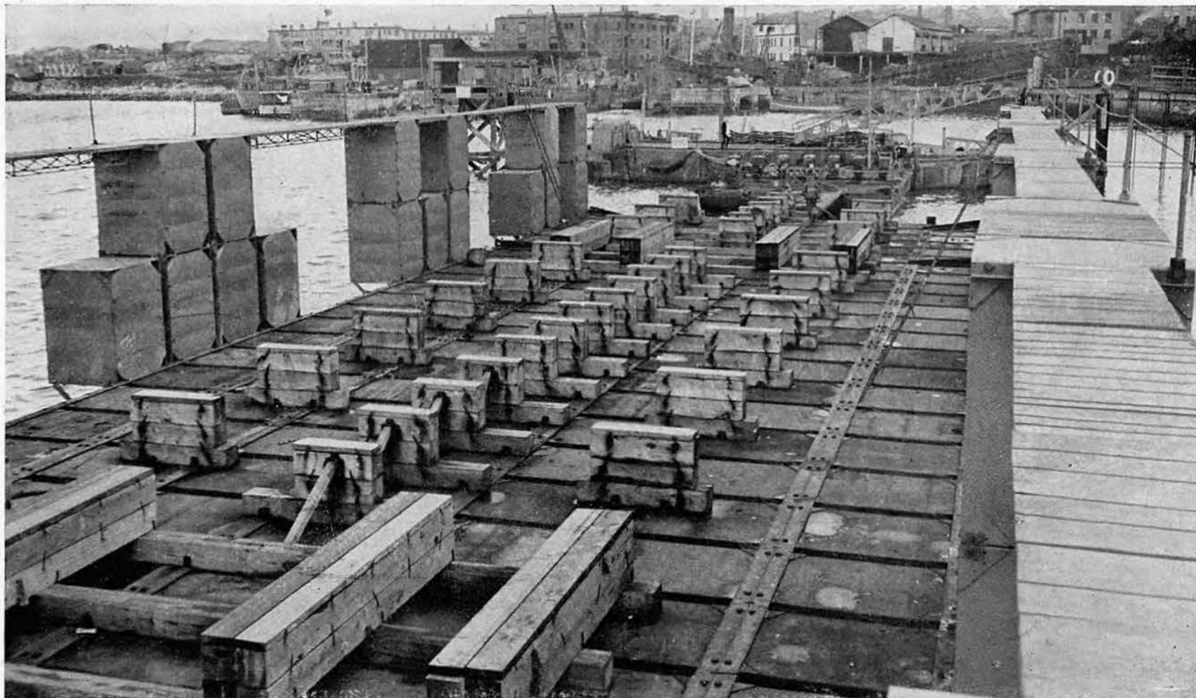
VIEW OF DRY DOCK with chocking partially installed, for receiving a vessel to be raised. The stabilizers maintain the deck in level position as it is sunken by water ballast let into the pontoons.
