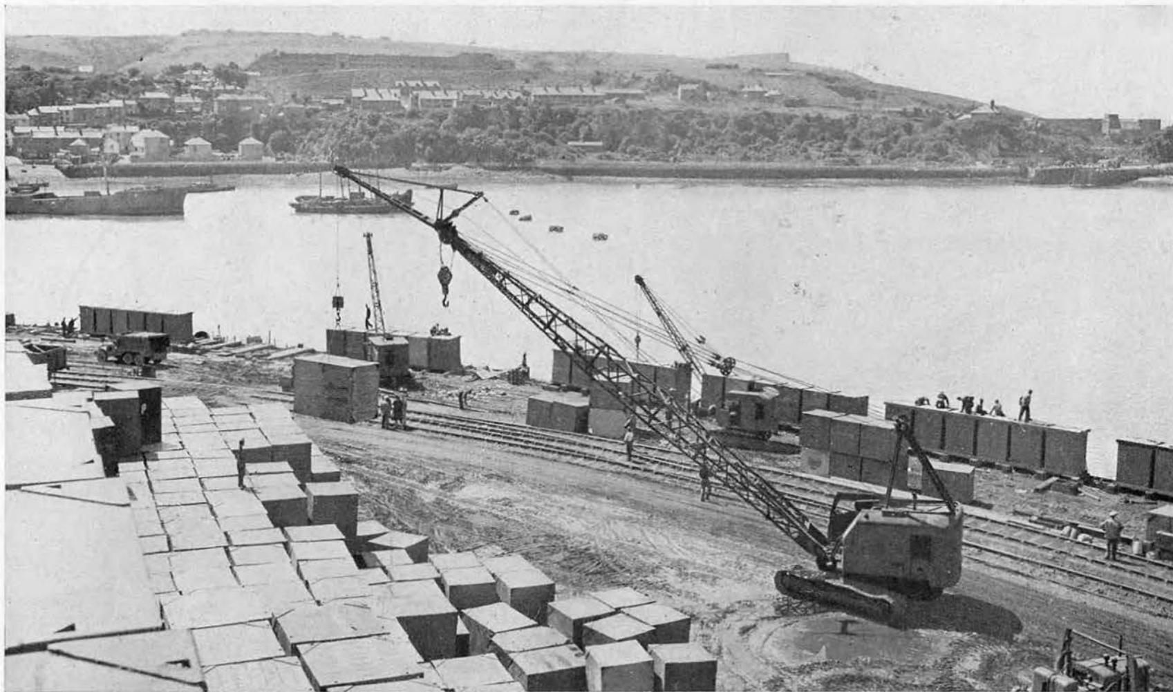
PONTOONS IN STORAGE STACKS, too high to be removed by smaller rigs, are lowered and distributed to within easy reach by a heavy crane with an eighty-five foot boom and jib.
