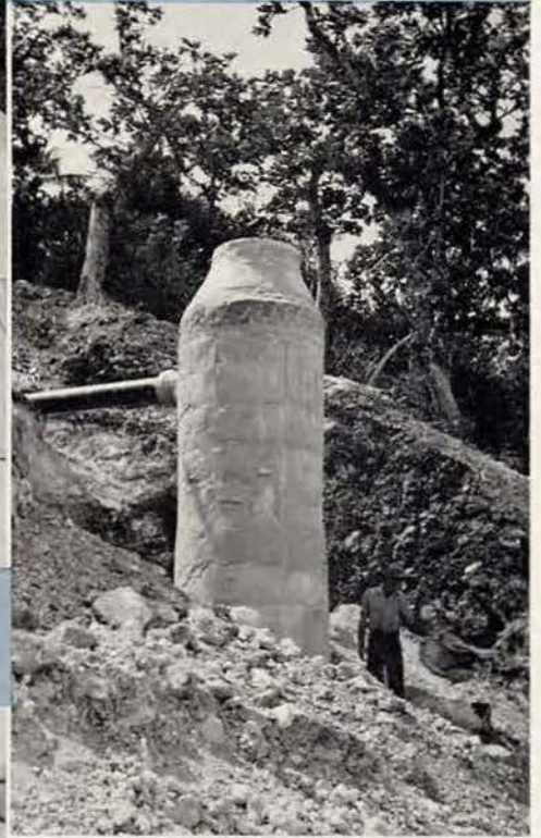
Concrete brick manhole in outfall sewer line. Manhole was exposed because of sharp drop of grade.
