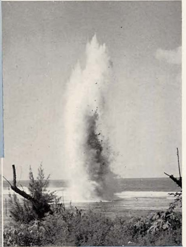
Underwater blasting of coral reef for outfall sewer, part of big Marianas Navy Administration Center project.
