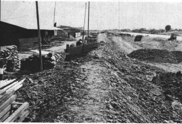
BERM BUILDING —Earthen berm shown under construction is typical of fortifications at Special Forces camps.
